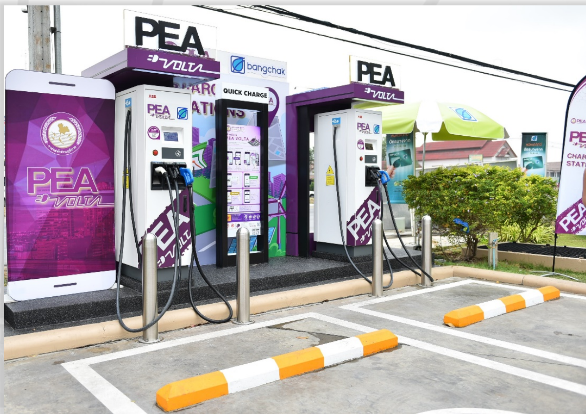
Exhibit 5: Example of Public EV Charging station in Thailand
